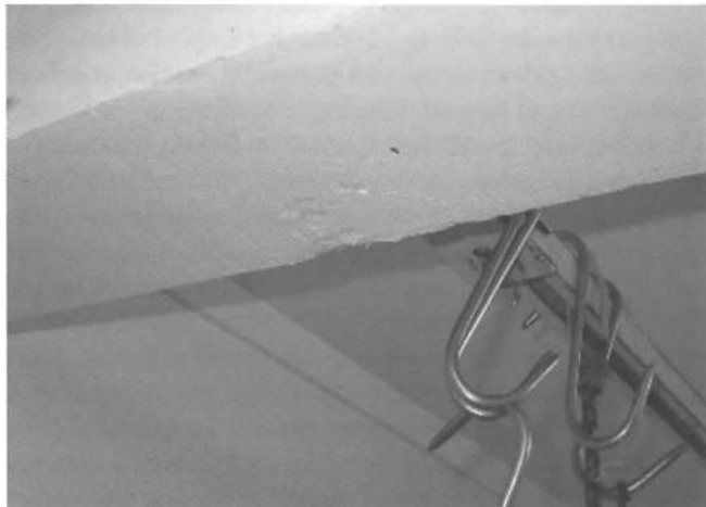
Worn plaster and steel painted tiebar.
