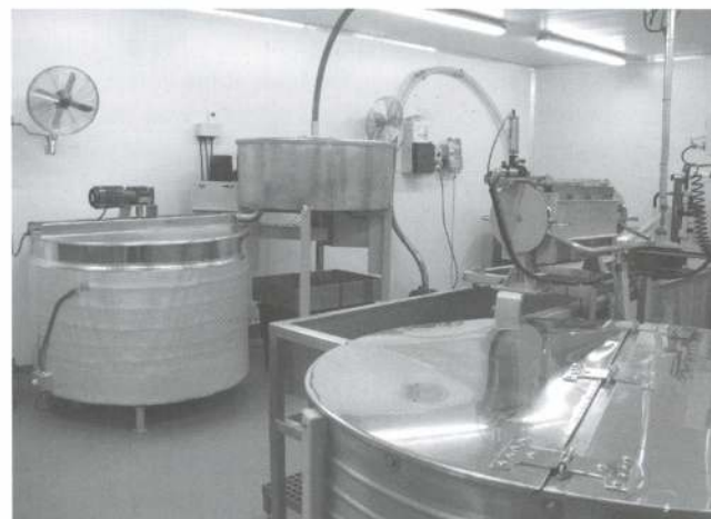
Spin float and storage tank (note the heat ribbon covered with foil on the tank).
