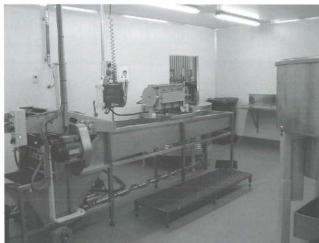
The floor is sealed with "easy flow" which is used in most freezing works as it is hard wearing.
